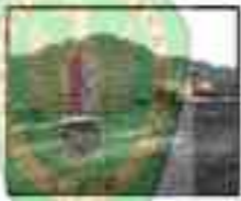
Figure 13. A pothole on the road.
